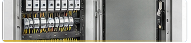
Koruma & RTU/SCADA Panosu Protection & RTU/SCADA Panel
